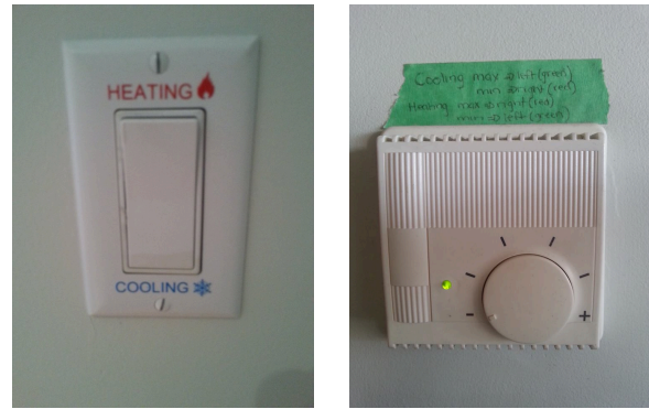
Figure 1. The Building 2 H/C controls
